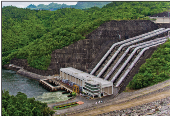
A hydropower station was experiencing low packing life when sealing a 25" turbine shaft.
